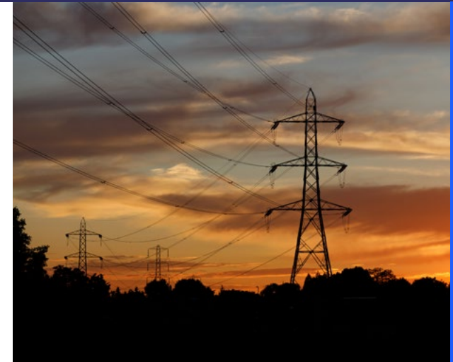
An electricity pylon
